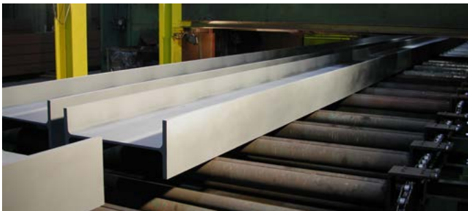
Automatic shot blasting to grades Sa 2.5 or Sa 3.0 and application of shopprimer
