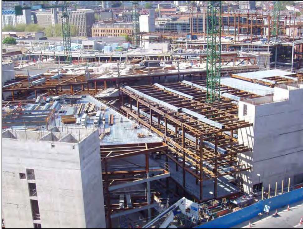
Figure 2.1 Rapid installation of steelwork and steel decking speeds up the construction process
